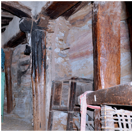
Fig. 5: Däbrä Zäyt, southern wall (the old mānbärä tabot is in the centre)
